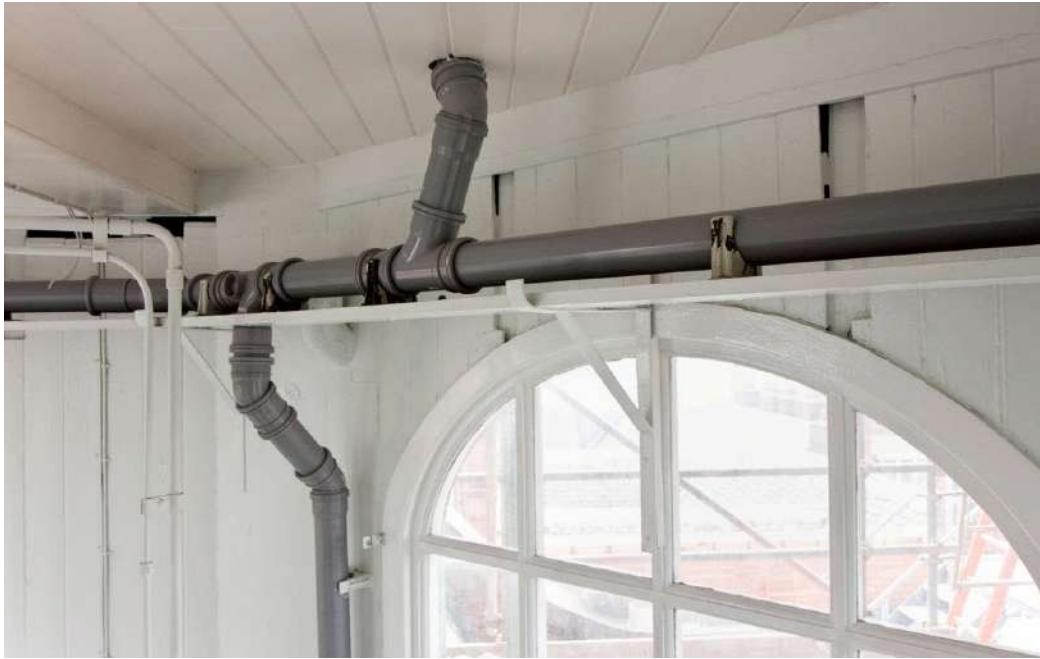
Pipes within Octagon room
